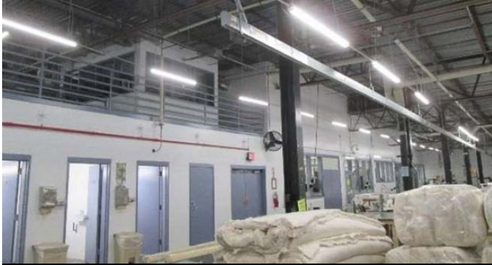
NECX laundry area with new LED lighting
