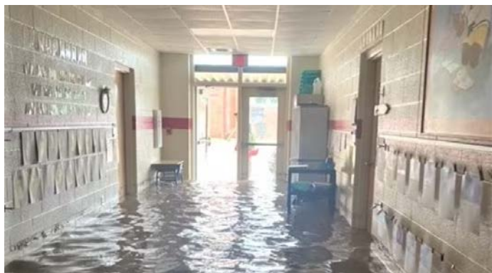
Flooding in the hallway of Waverly Elementary School.
