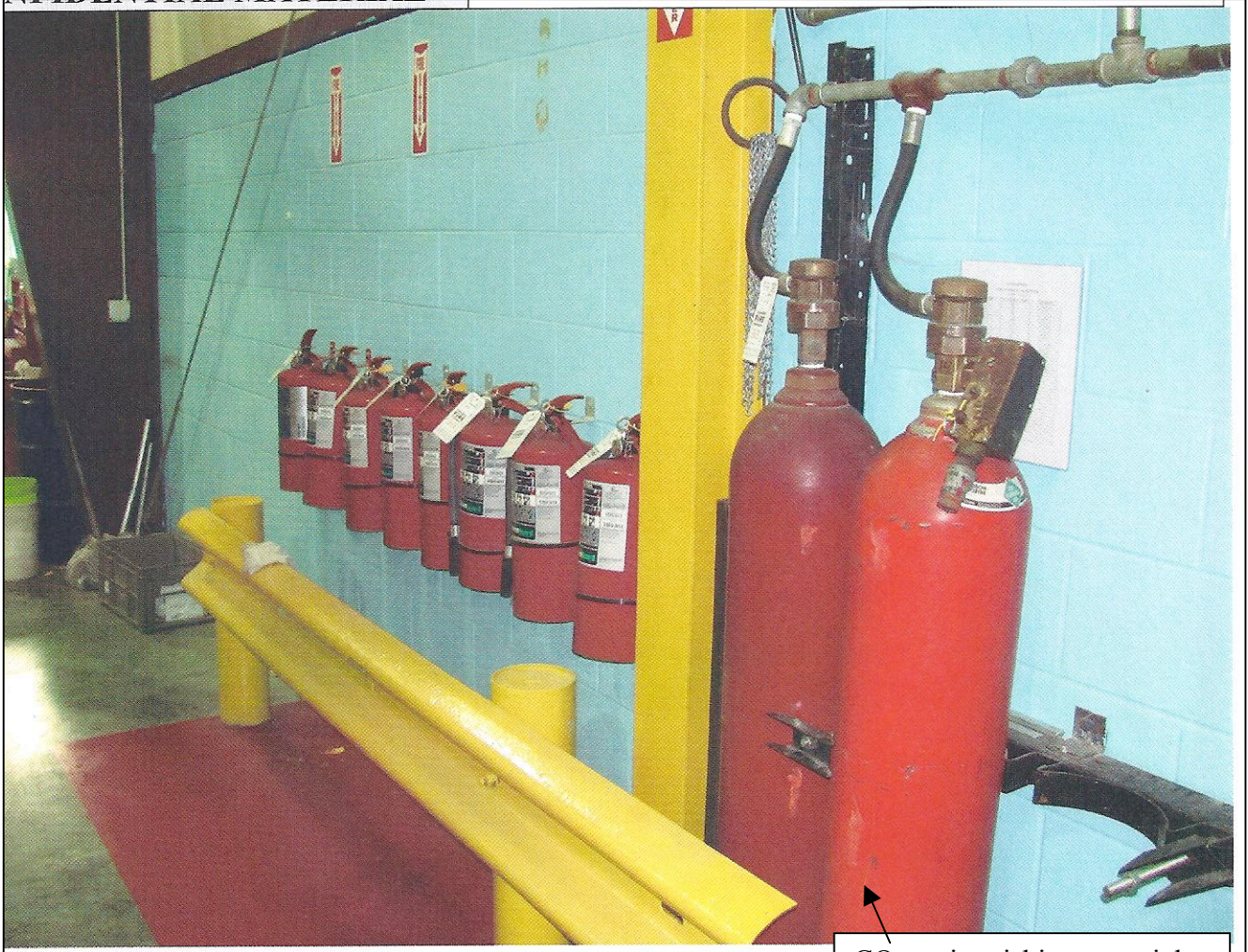
CO 2 extinguishing material
