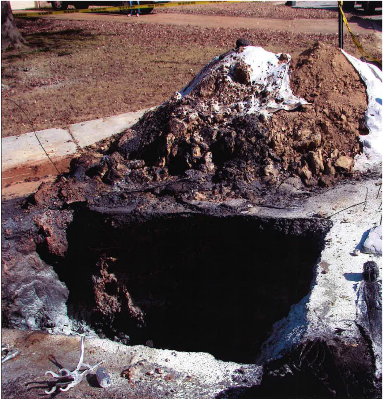
Photo 1 of 1: Natural gas explosion
