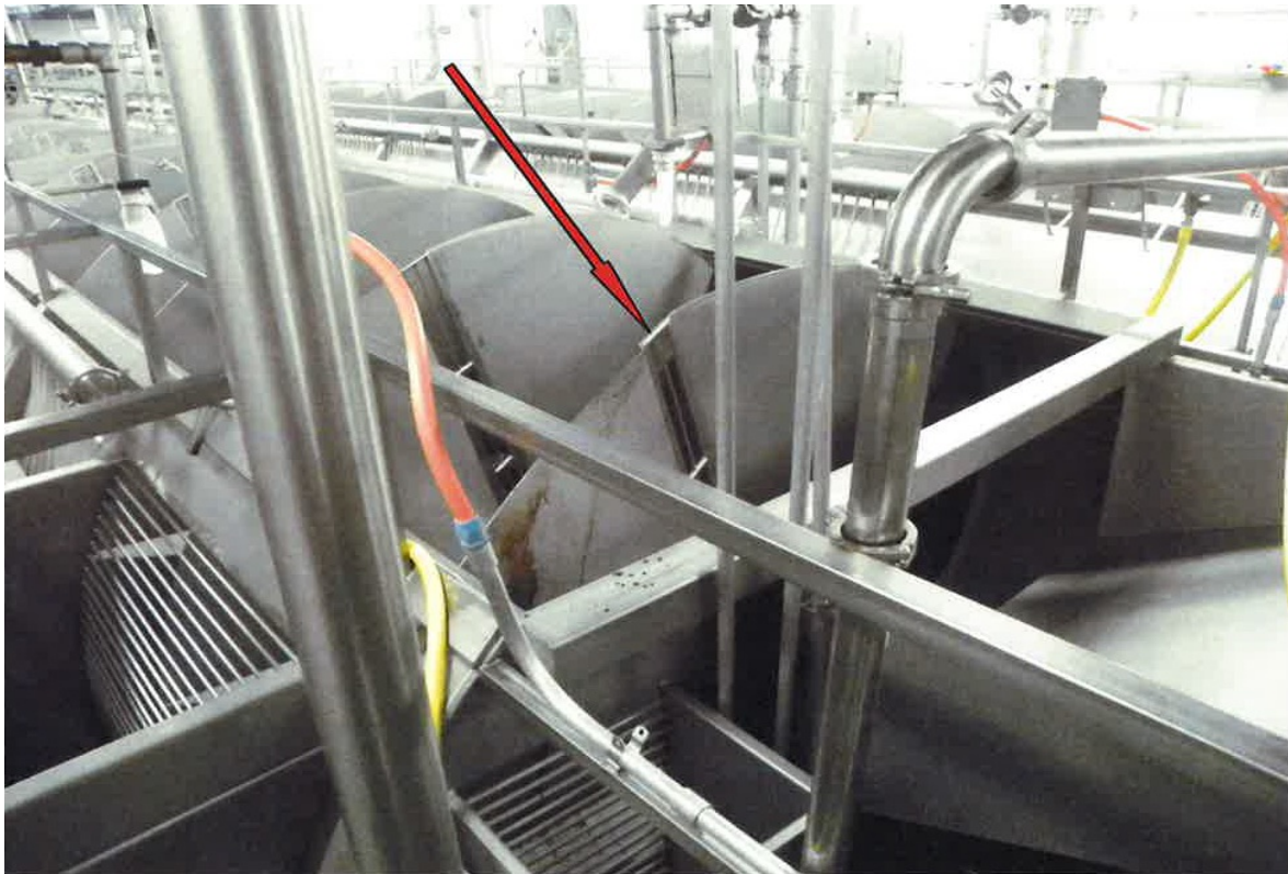
Photo 1 of 1 – Photograph showing the auger in chiller #2
