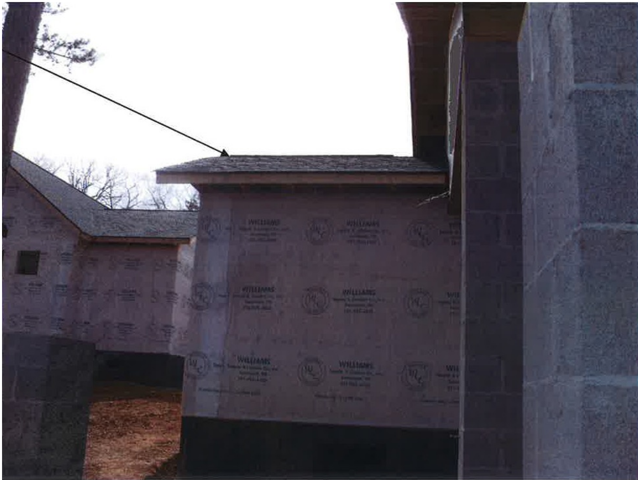
Photo 1 of 2 – Photograph showing the roof that the victim fell from.
