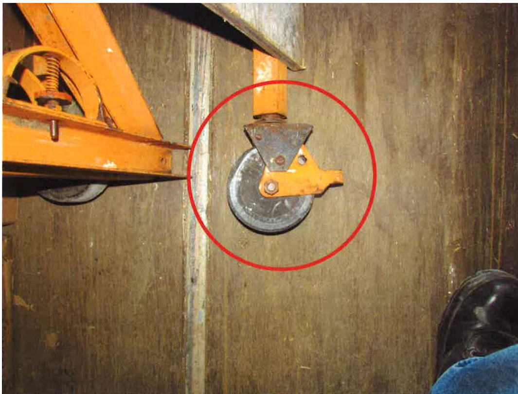
Photo 1 of 1 – Caster/wheel lock from the baker-style scaffold (engaged) in position to prevent movement of the scaffold wheel. The scaffold wheel was able to spin freely when the lock was engaged.
