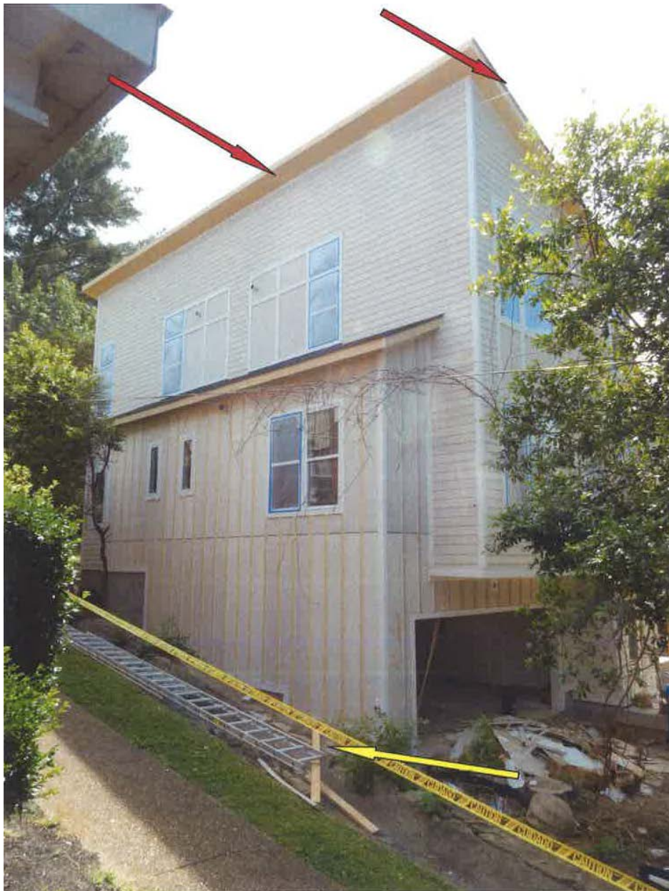
Photo 1 of 1 – West side of the house where the employees contacted the power line (red arrows) with the 40 foot aluminum ladder (yellow arrow).
