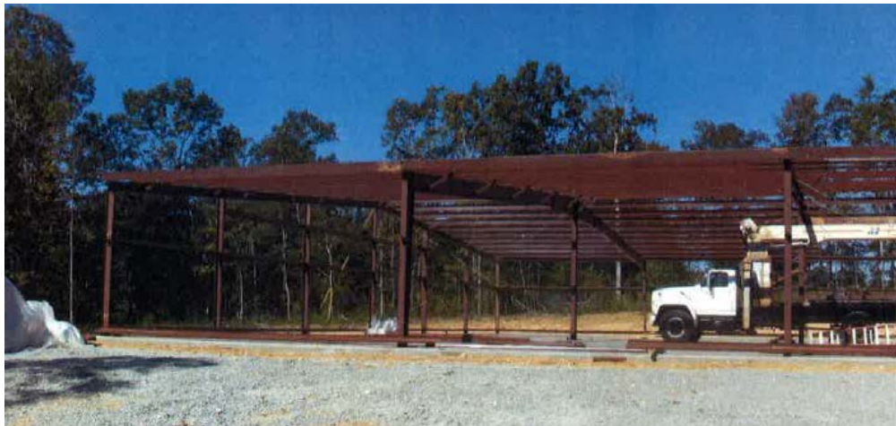
Photo 1 of 1 – Photo shows a view of the steel building where the employees were working the incident occurred.
