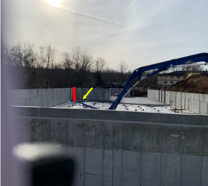
44 Struck by concrete truck boom—Insp # 1506283 HC Concrete Construction
