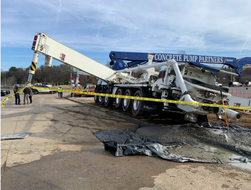
44 Struck by concrete truck boom—Insp # 1506283 HC Concrete Construction
