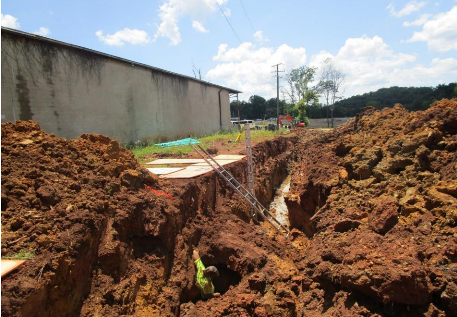
21 Crushed by cave-in—Insp # 1682055 Design One Building Systems, Inc.
