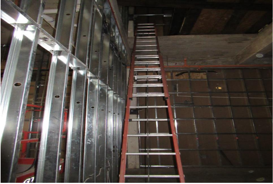
Fall from ladder—Insp # 1696251 Ryno Construction, LLC
