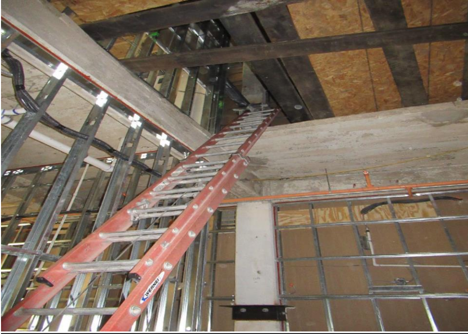
Fall from ladder—Insp # 1696251 Ryno Construction, LLC
