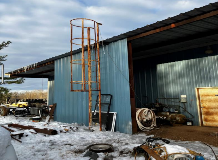
10 Fall through skylight—Insp #1721951 Big G Metal Works Inc.
